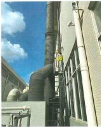
处理后废气采样
